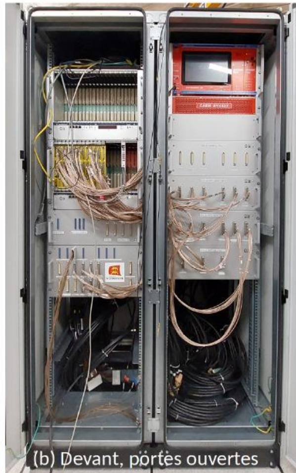
Front view opened doors
